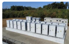
Iwate Kitakami Power Storage Station, a grid storage operated by Tokyo Century
